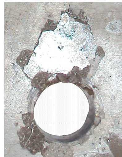
Figure 5.96: Example of bearing failure
