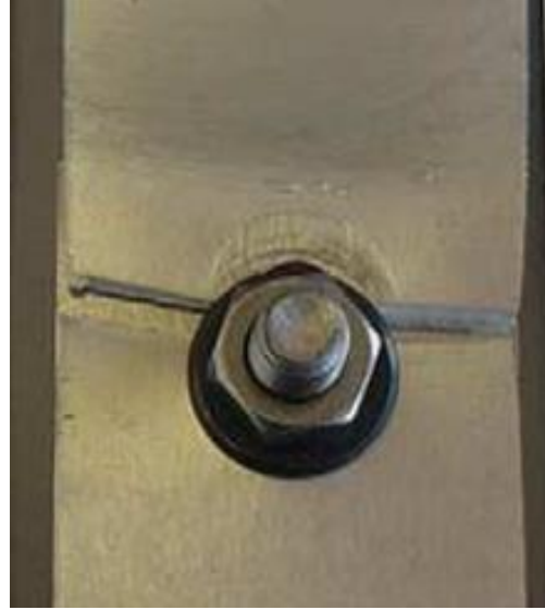
Figure 5.8: Failure on steel plate
