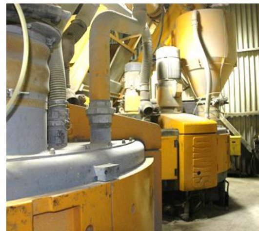
Figure 3.23: General view of the mixer
