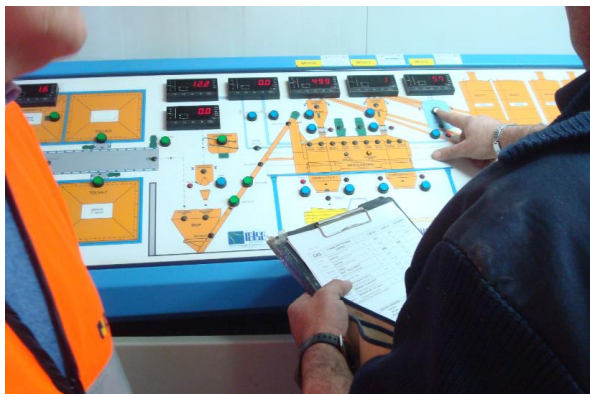
Figure 3.20: Control panel of the industrial mixer
