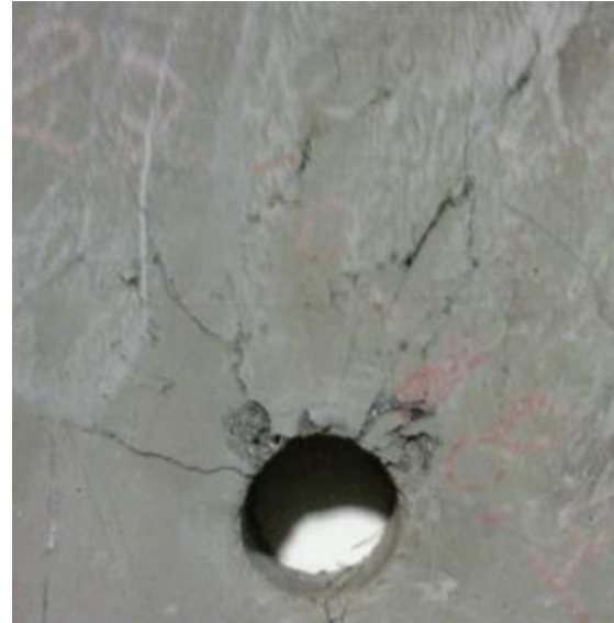
Figure 5.18: Bearing failure mode
