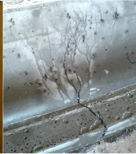
Figure 3.39: Crack in the center of the span of the prestressed beam
