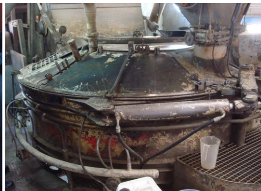
Figure 3.21: General view of the mixer
