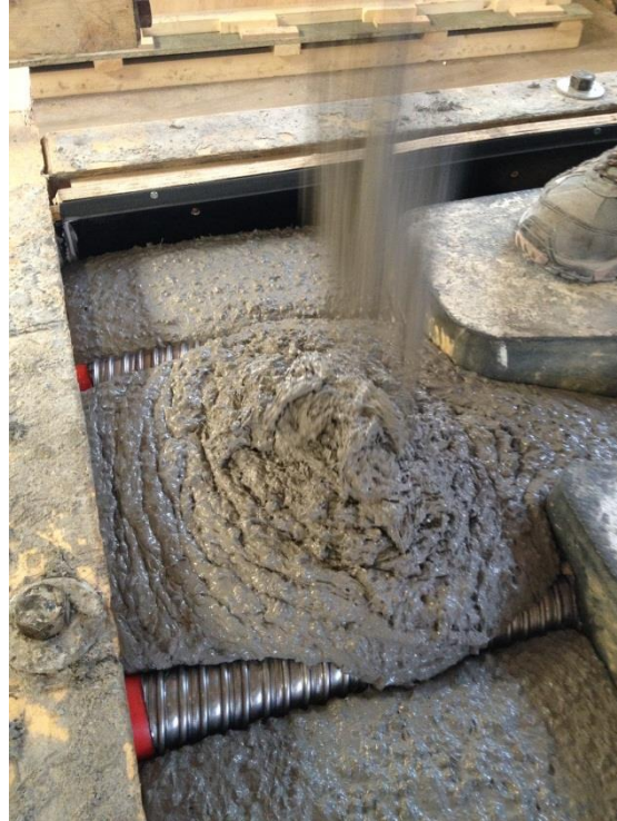
Figure 5: Low w/c ratio makes the concrete thixotropic
