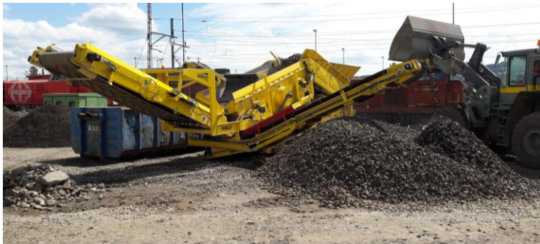
Gravel cleaning , in-situ or with mobile cleaning system. Share of ballast cleaning must increase due to scarce availability.
