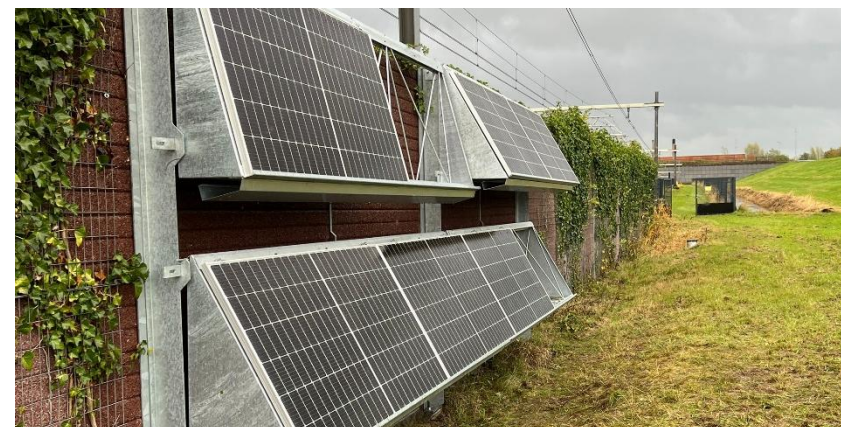
PV-LSW in Holland (ProRail)
