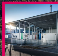
Energy System Integration
