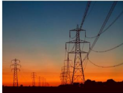
The power is carried by aluminum wires, suspended by glass, polymer, or porcelain insulators.
