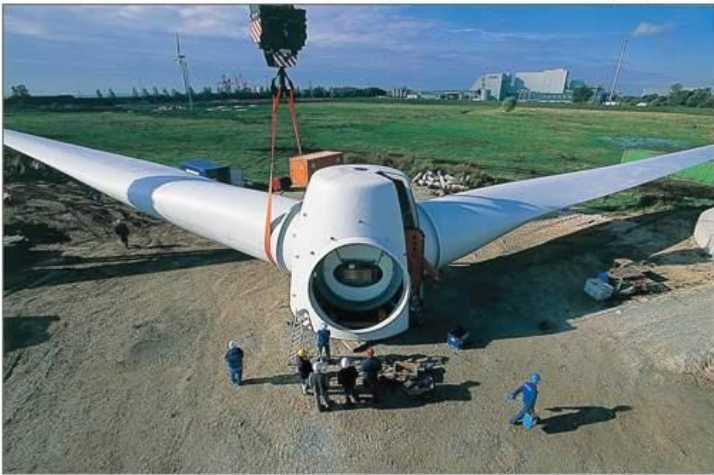
A close up view of the rotor as it awaits installation of its third 61.5m blade. Source: LM Glasfiber
