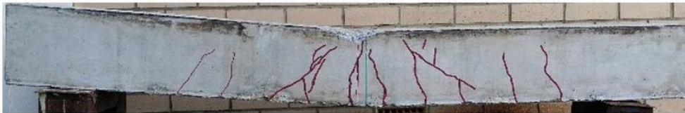
Failure under impact load
