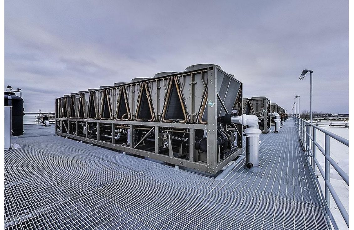
Condenser in Cooling Systems, STACK
