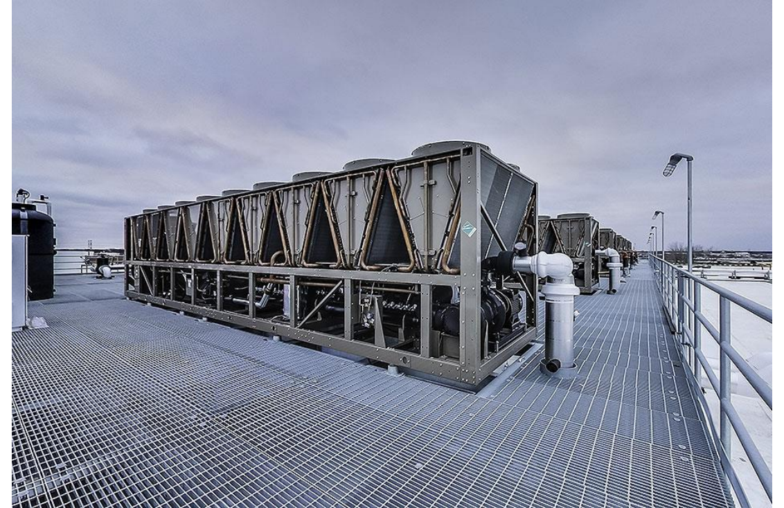
Condenser in Cooling Systems, STACK
