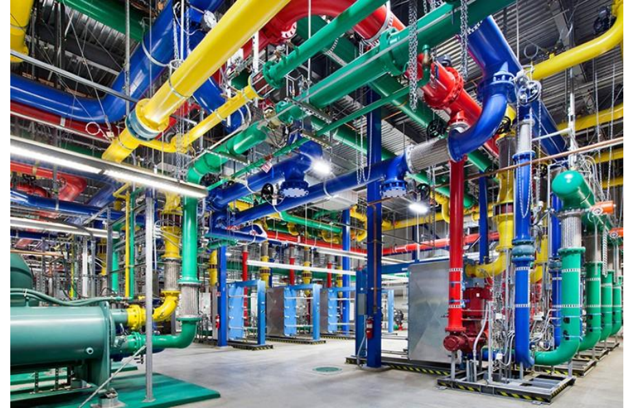
Cooling pipes in a Google data center (Credit: Connie Zhou/Google/Zuma)
