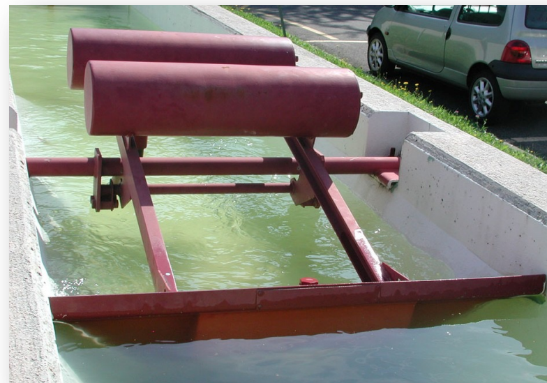
The AMIL hydromechanical gate installed in the network
