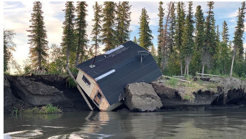
Infrastructure in permafrost areas is threatened by riverbank erosion, Mackenzie River Delta, Canada.
