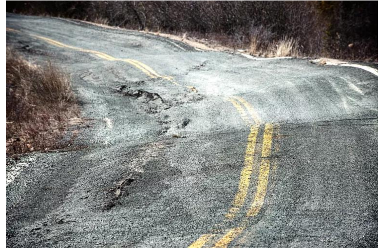
Effects of global warming as the permafrost thaws near Yellowknife in Canada's Northwest territories. The pavement is buckled and pot-holed.
