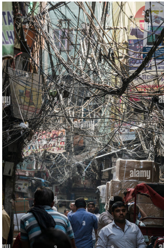
Figure 23.1: Electric cabling above a street elsewhere where they don't read this manual. The cabling in your project will likely look similar unless you consciously do something about it.
