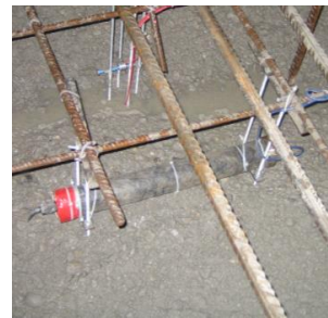
c) final application of the filled and closed stressmeter and continuation of casting
