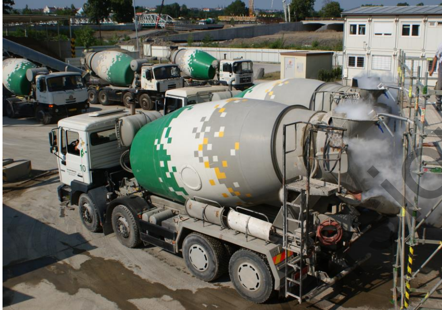
Fig. 6.1 Photo of typical in-site application of LN cooling in concrete truck (courtesy of O. Kunc, TBG Metrostav)
