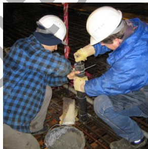
b) filling and compacting of the tube with fresh concrete when casting reaches the measurement point
