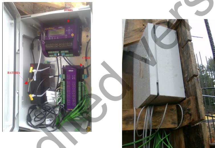
(a) Data logger and battery inside the box (b) Impermeable electric box with data logger inside
