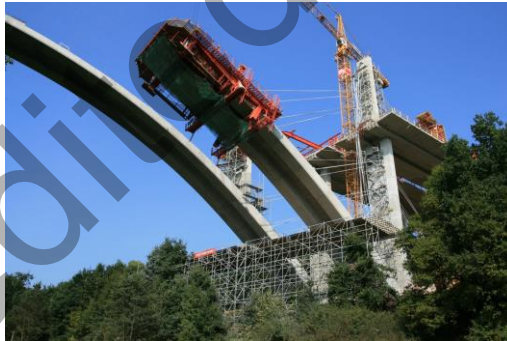
Fig. 7.6 Two arches of Oparno Bridge during construction (Photo by Jan L. Vitek)
