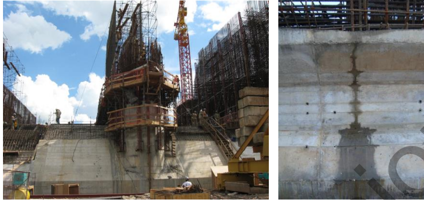
Fig 1.4 Spillway of small hydropower plant and thermal cracking. ( Funahashi Jr and Kuperman, 2010)
