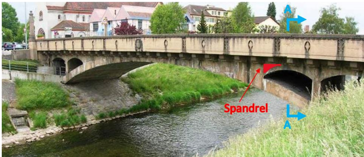
Figure 1: Guillermaux bridge showing geometry and existing condition
