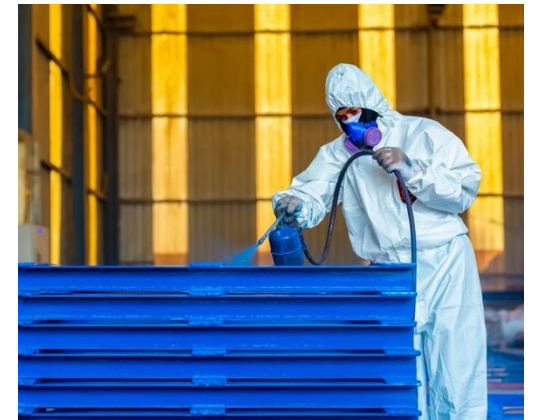
Corrosion and metal protection
