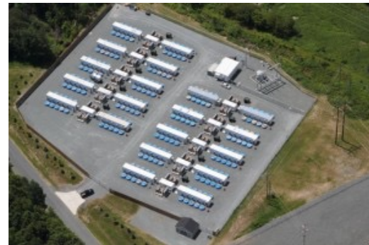
station de stockage
