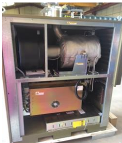
Containerised Capstone C30 Micro-turbine
