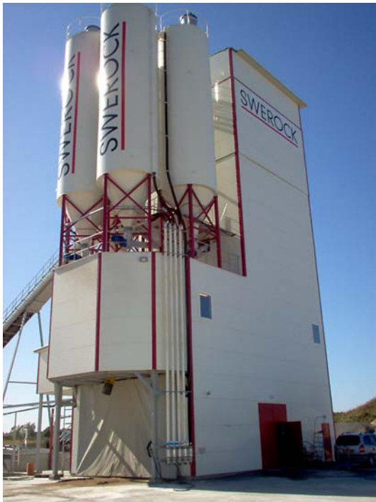
Fig. 4 A modern concrete mixing plant with several silos (Courtesy of Swerock, Sweden)
