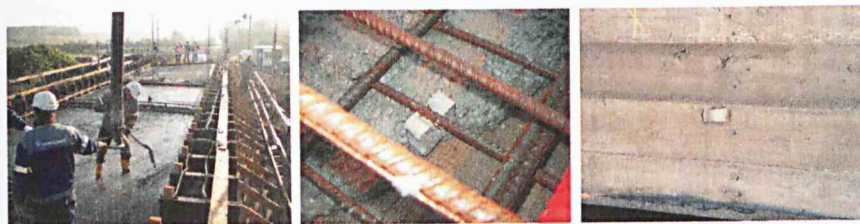
Figure 10.6 Small SCC bridge over motorway at Give, Denmark. Left: Casting and finishing of bridge deck. Mid and right: Examples of casting and improper compaction around spacers. SCC, Self-compacting concrete.
