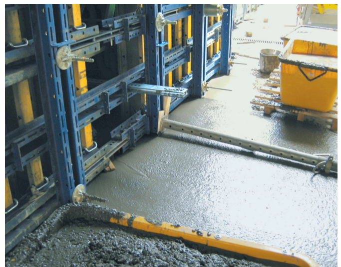
Fig. 10. Damage on a construction site: the formwork was inadequately designed and constructed and so did not bear up to the pressure of fresh concrete!
