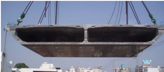
Photo 5 Cross section of girder
