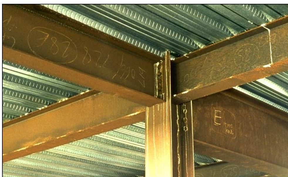
Figure 1-2 View of unprotected steel structure
