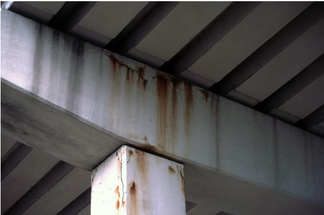
Figure 2 Rust stains and cracking in bridge cross beam due to reinforcement corrosion
