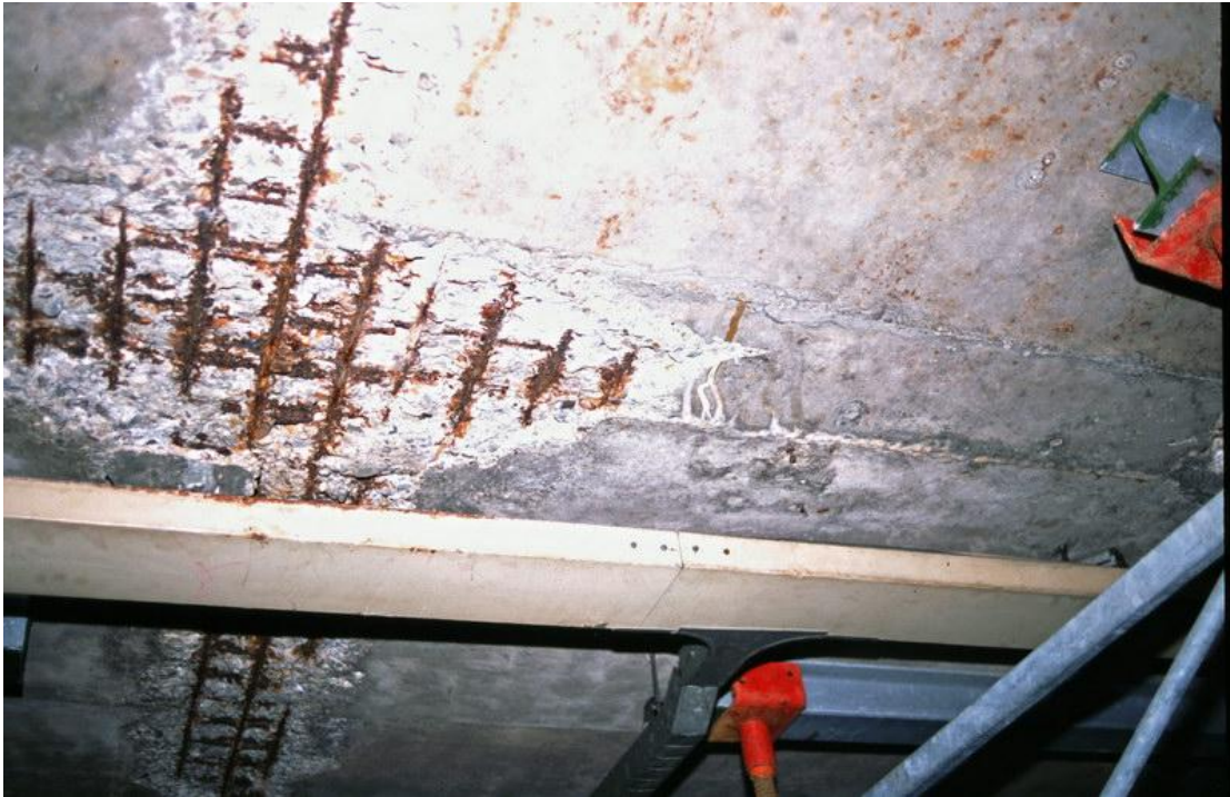
Figure 3 Spalling and delamination due to corrosion
