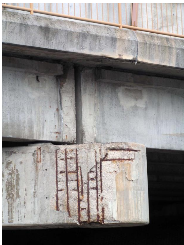
Figure B.5 Reinforcement corrosion and concrete spalling
