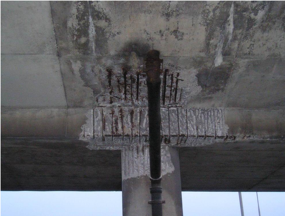
Figure A.1.4 Corrosion damage due to leaking drain system in motorway bridge near Warsaw
