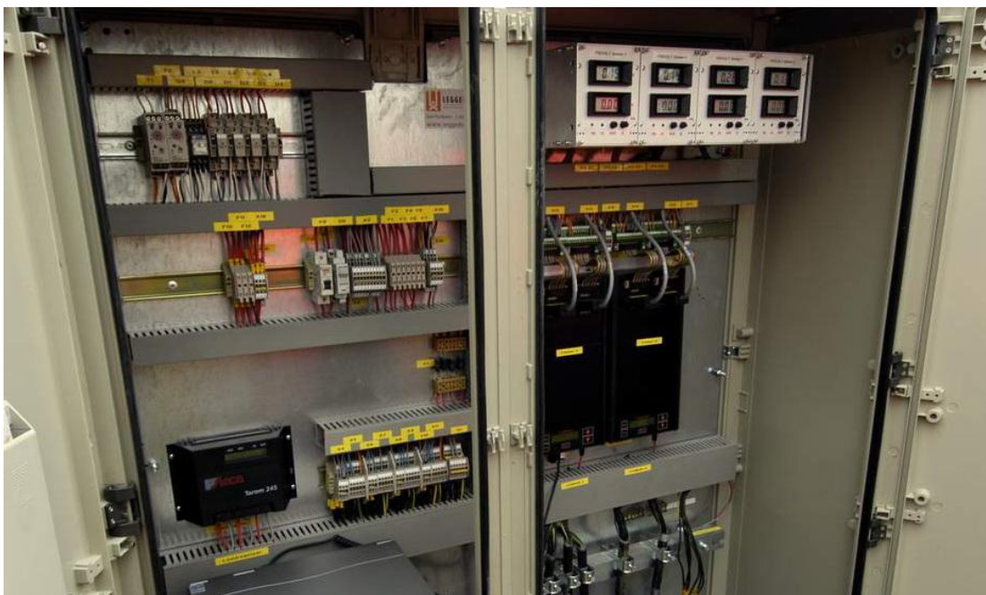
Figure 9 CP system control box with four power units (top right), datalogger/remote control (middle right), cable connections and testing points (left)
