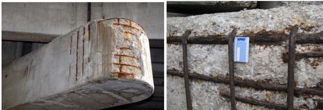
Figure A.1.1: The damaged bridge substructure in Slovenia
